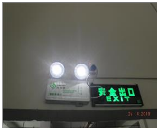
External photo(s) of the production unit(s) Emergency lighting testing.JPG
