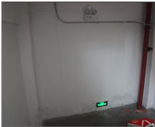
External photo(s) of the production unit(s) Corrective action taken for 7-15 emergency light and evacuation sign in staircase.JPG
