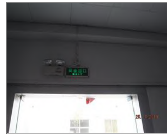
External photo(s) of the production unit(s) Safety exit sign and emergency light.JPG
