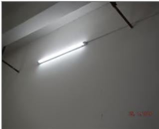
External photo(s) of the production unit(s) 7-7 Not explosive-protected lighting in chemical warehouse.JPG
